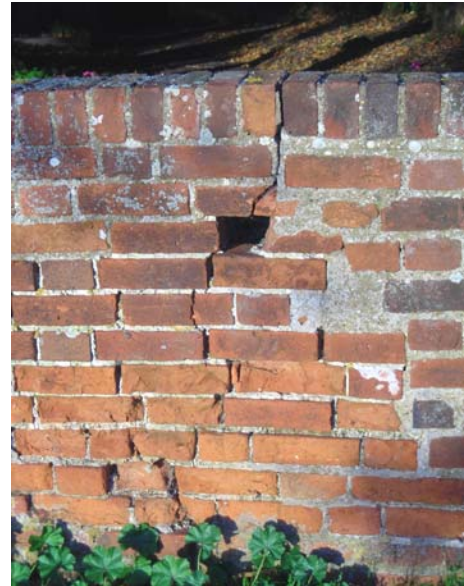
Fig. 34 Cracking, churchyard boundary wall, south side.
