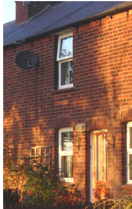
Fig. 35 Replacement UPVC windows and satellite dish, Brick Row.
