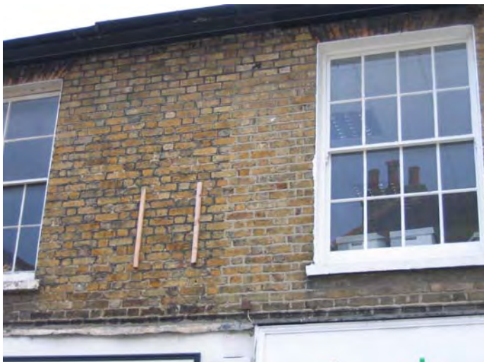
Fig 12 Nos 21-23 west Street. To the left, stock brickwork with tuck pointing. To the right, unnecessary repointing has had an adverse effect on the character of the brickwork.
